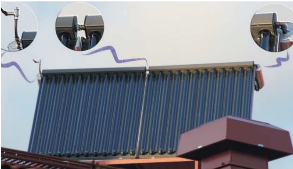
The solar collectors on the school roof are a part of the educational unit.
