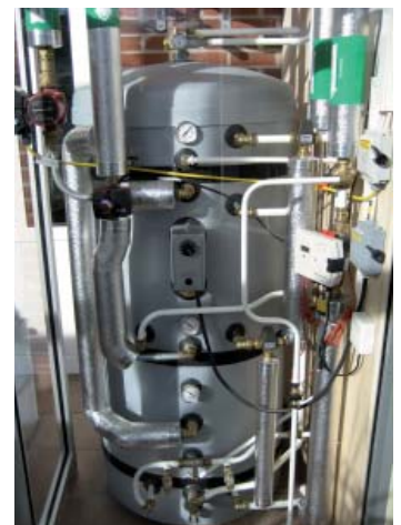
The accumulator tank.
